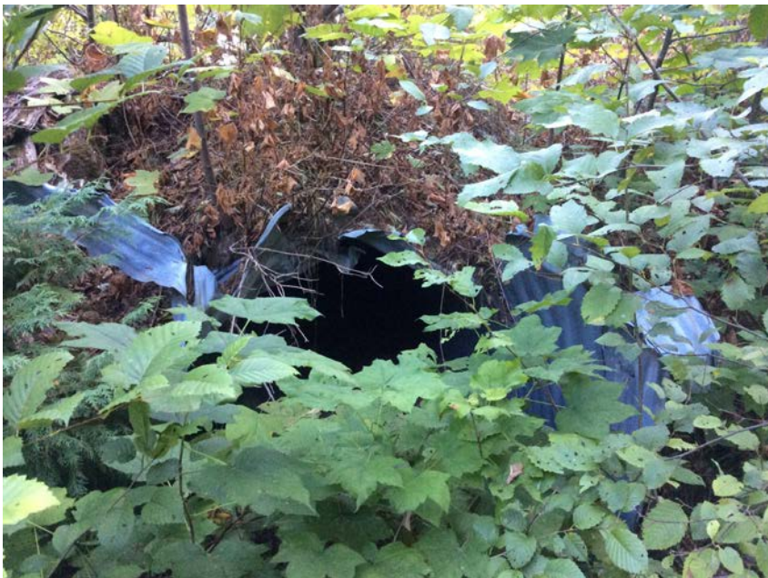
Damaged inlet likely from excavator cleaning bedload
